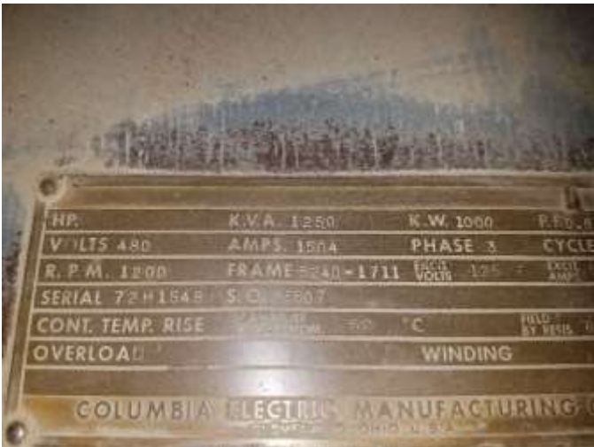
106. Serial plates 3 different 1000 Kw generators
