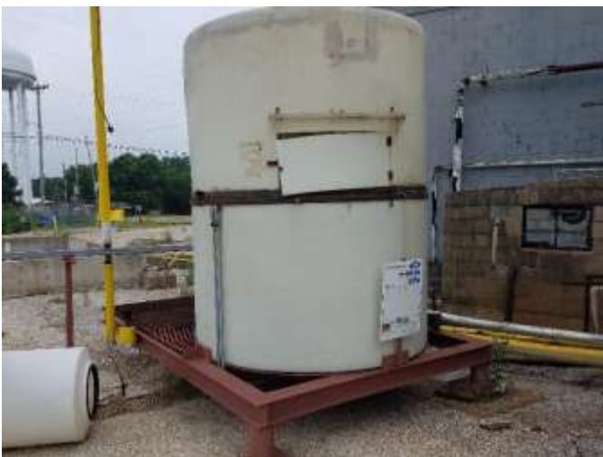
190. Ashland chemical storage tank 500 gallon
