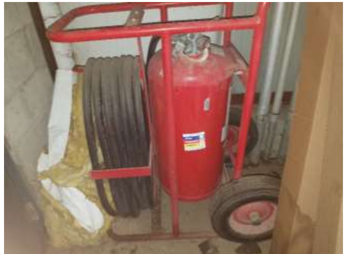
30. 150 lb AMEX wheel fire extinguisher
