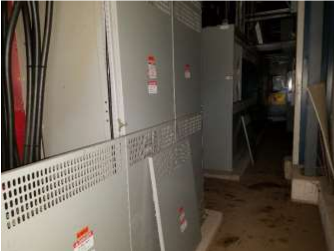
43. Control panel generator room
