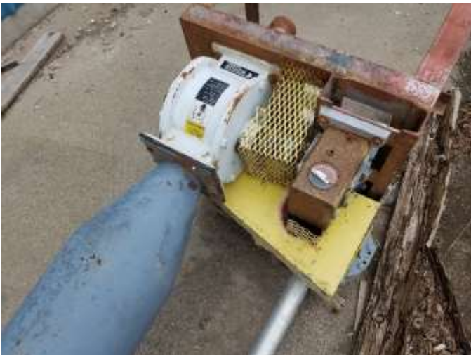
124. Gear box on auger
