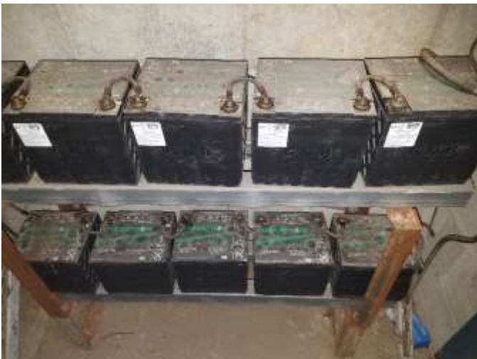
132. Inside control panel room
