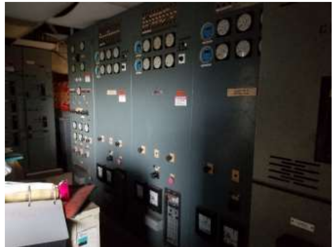
214. Generator control room
