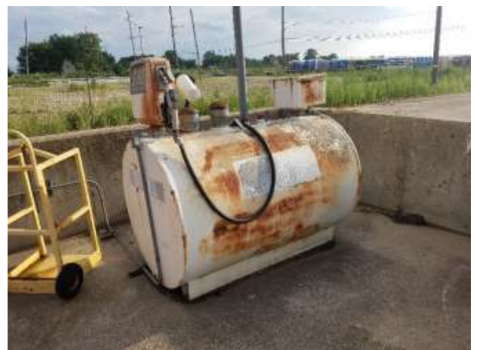
194. 500 gallon white fuel tank w/electrical pump (200 gallons in it)
