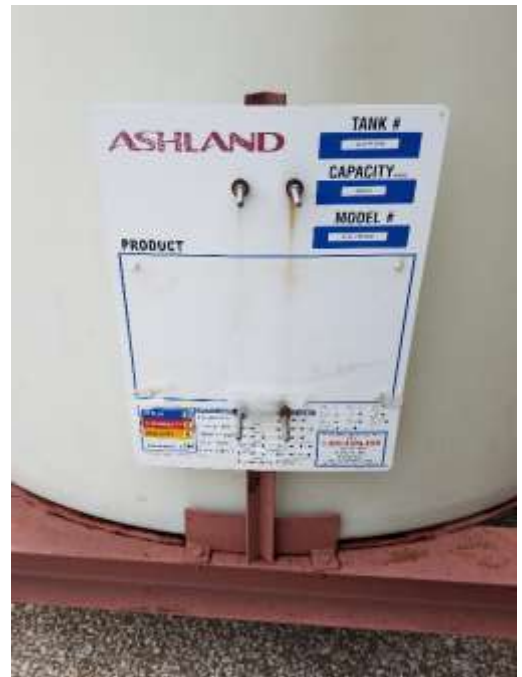
187. Ashland chemical storage tank 500 gallon
