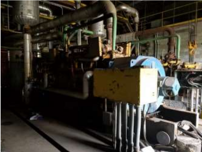
205. 1000 KW generator in generator room
