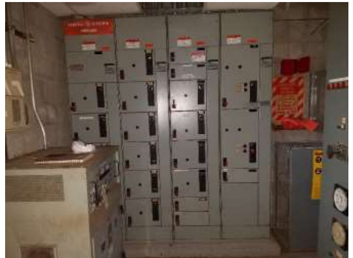
133. Inside control panel room
