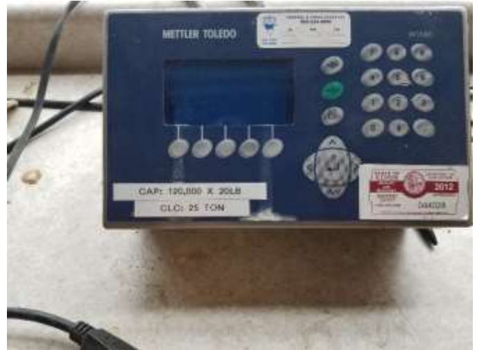
89. 90 foot truck scale equipment
