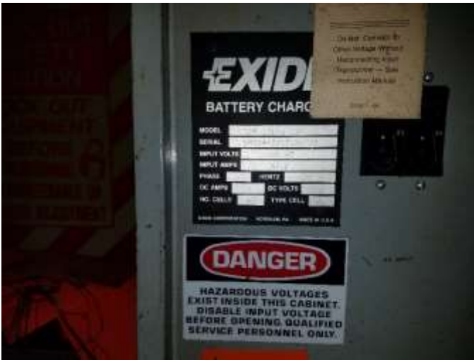
136. Inside control panel room
