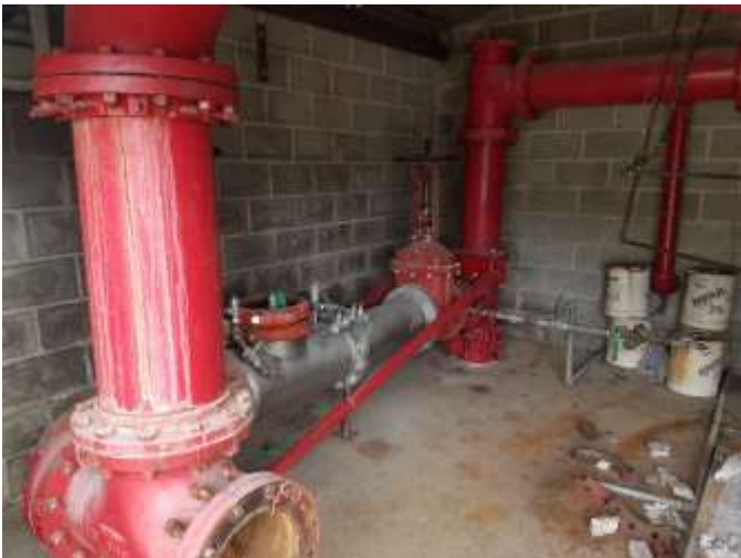
199. Sprinkler system equipment
