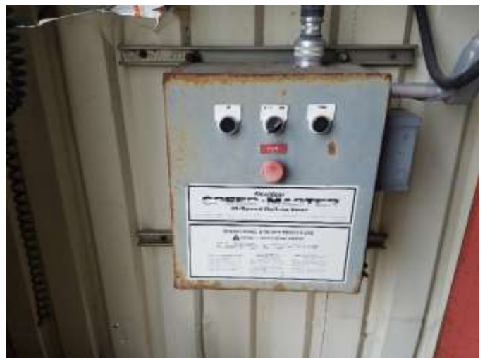
85. 90 foot truck scale equipment
