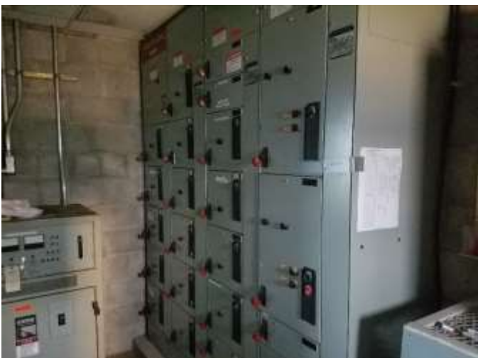
217. Generator control room
