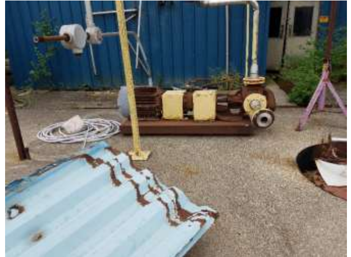
139. Vacuum pump with motors
