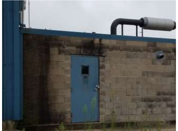
115. Outside large generator room
