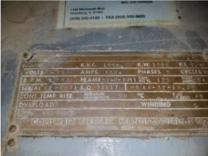
104. Serial plates 3 different 1000 Kw generators
