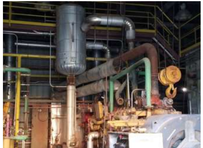
208. 1000 KW generator in generator room
