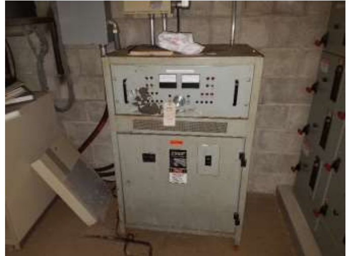
131. Inside control panel room
