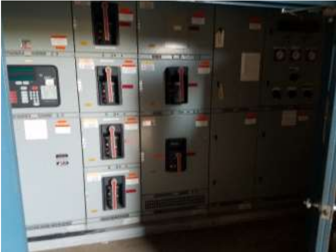
213. Generator control room
