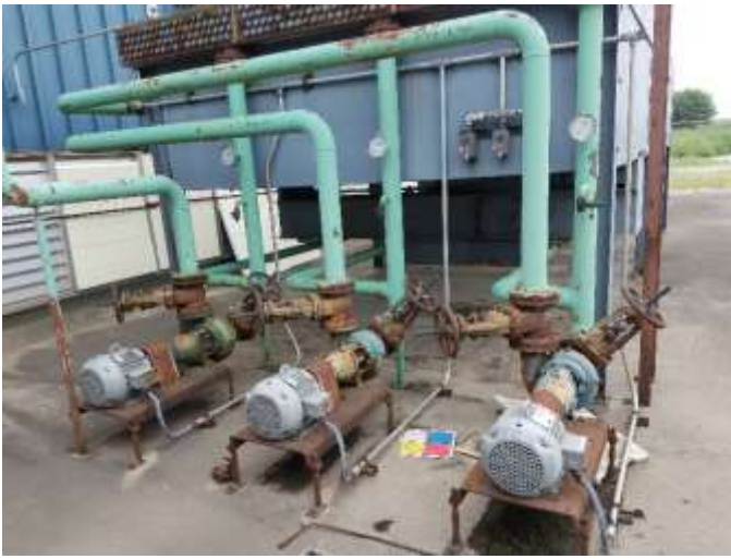
33. Cooling tower equipment
