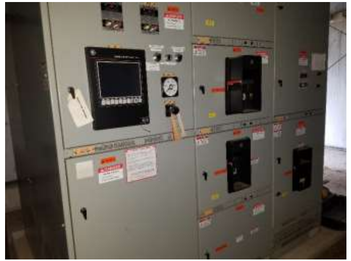
42. Control panel generator room
