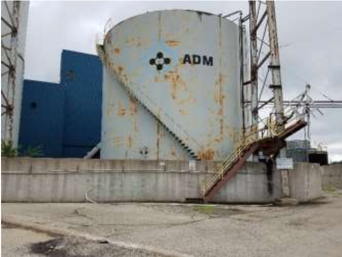
3. Soybean oil tank with stairs
