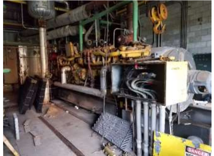
206. 1000 KW generator in generator room
