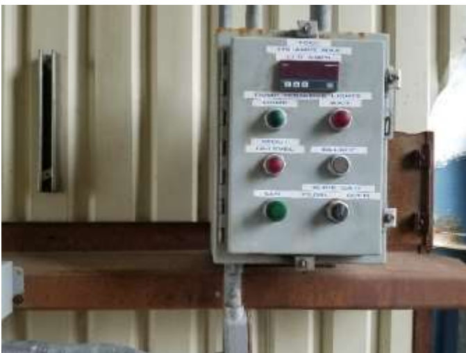
84. 90 foot truck scale equipment
