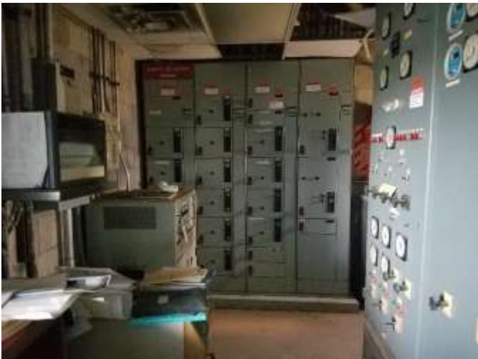
215. Generator control room
