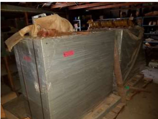
47. Parts inside far east building Includes 2 electric boilers never used
