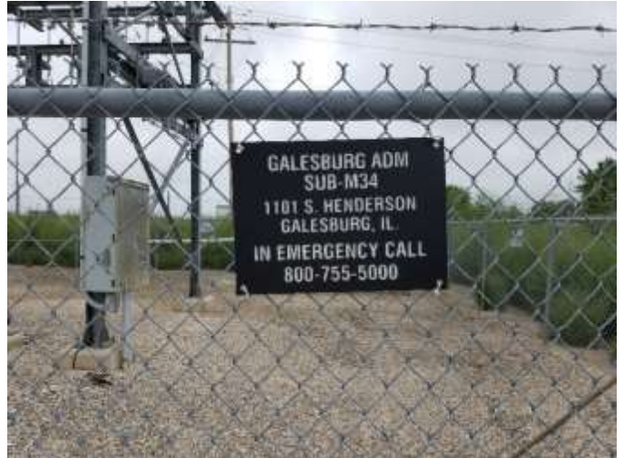
123. Transmission line (power into plant)
