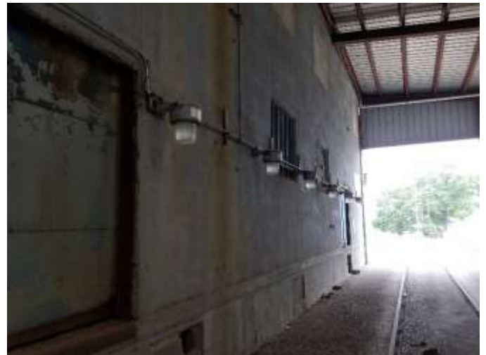
149. Outside security lights
