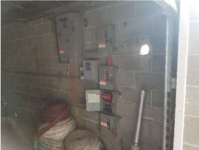
197. Fuse boxes, disconnects, control boxes
