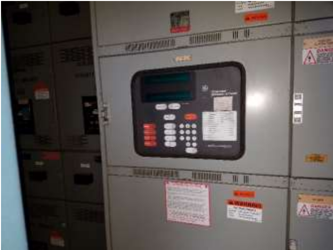
130. Inside control panel room
