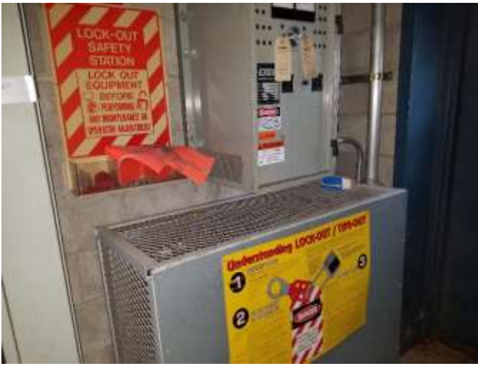
128. Inside control panel room
