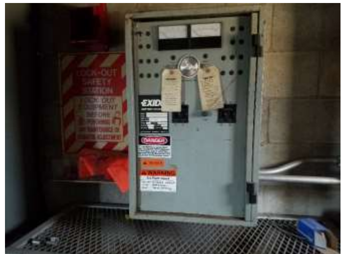
216. Generator control room
