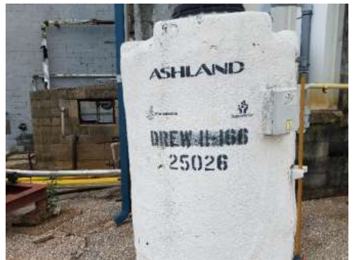
189. Ashland chemical storage tank 500 gallon
