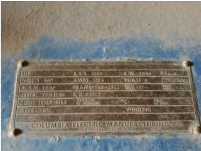
207. 1000 KW generator in generator room
