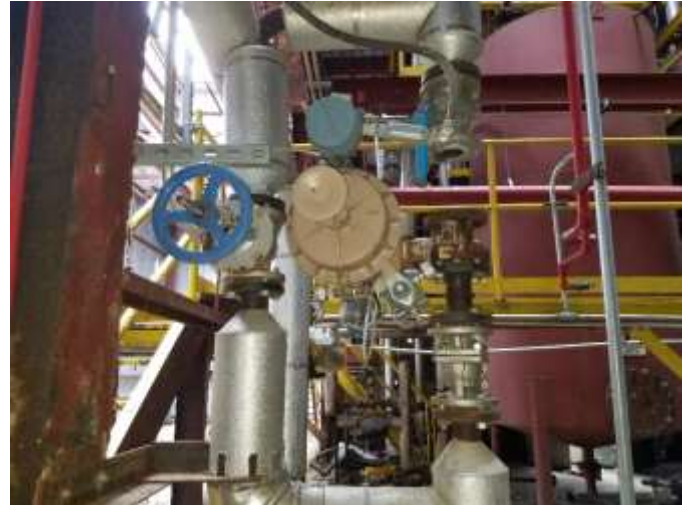
61. Processing valves & shutoffs
