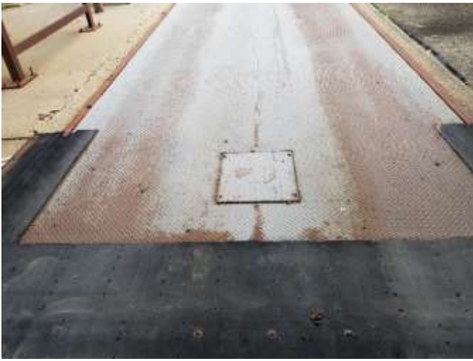
86. 90 foot truck scale equipment
