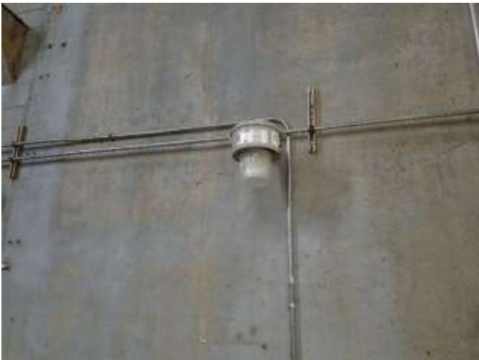
148. Outside security lights (17)
