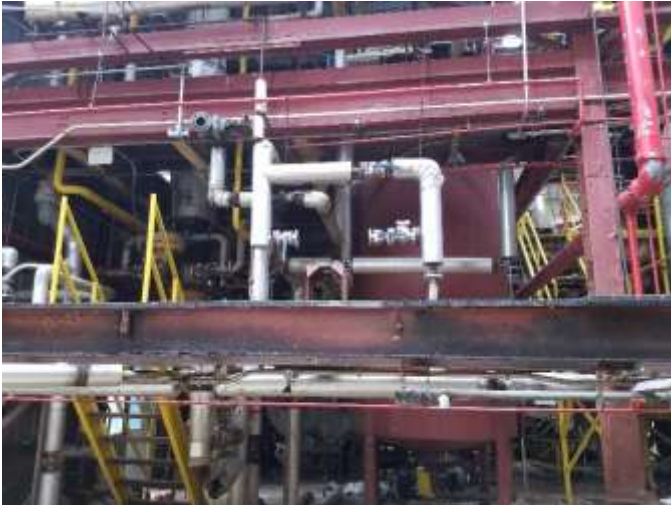
60. Processing valves & shutoffs
