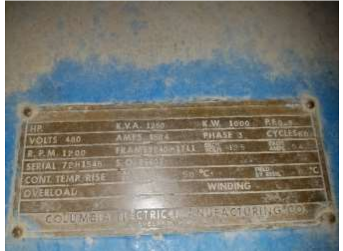
105. Serial plates 3 different 1000 Kw generators
