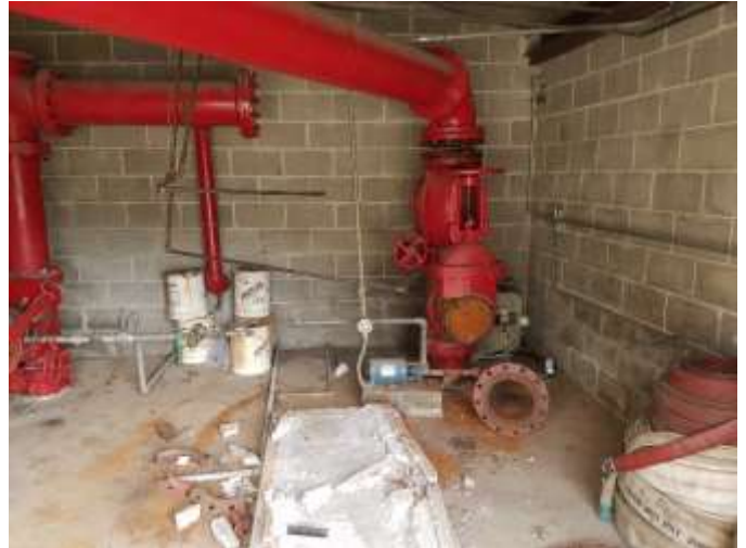
198. Sprinkler system equipment
