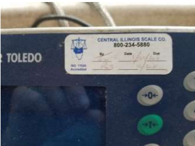
92. 90 foot truck scale equipment
