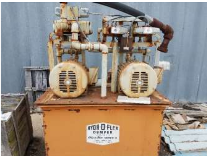
74. Large hydraulic unit
