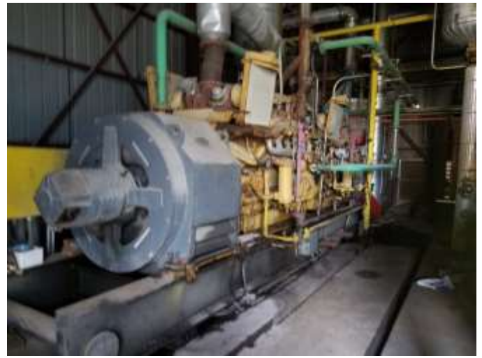
204. 1000 KW generator in generator room
