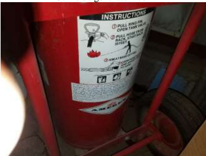
31. 150 lb AMEX wheel fire extinguisher
