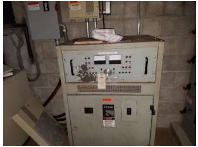
137. Inside control panel room
