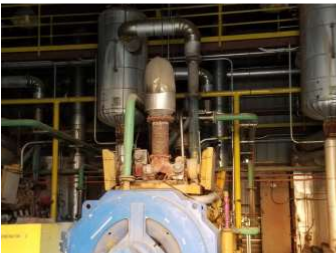
209. 1000 KW generator in generator room
