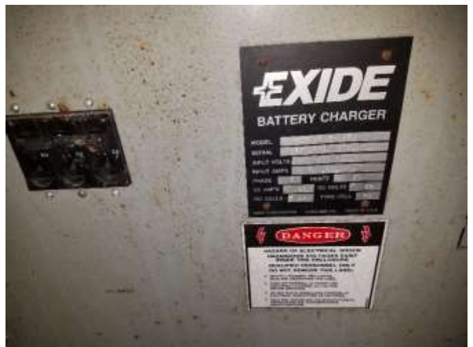
127. Inside control panel room
