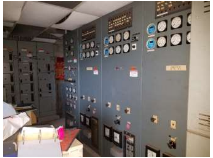
129. Inside control panel room
