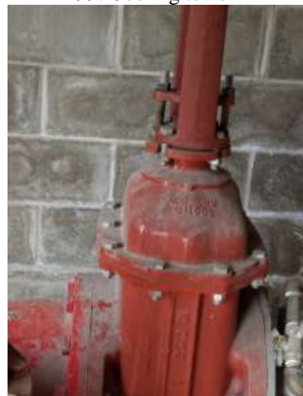
101. Sprinkler system valve
