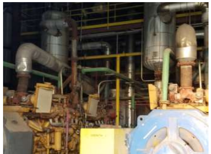
210. 1000 KW generator in generator room
