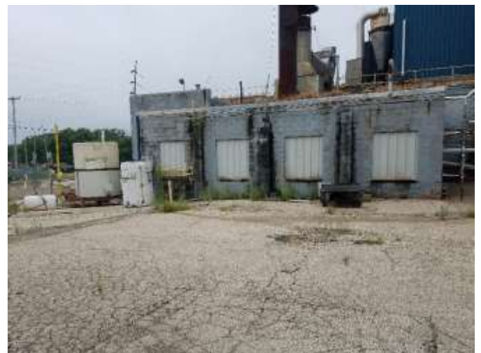
192. Overhead garage doors 10'
