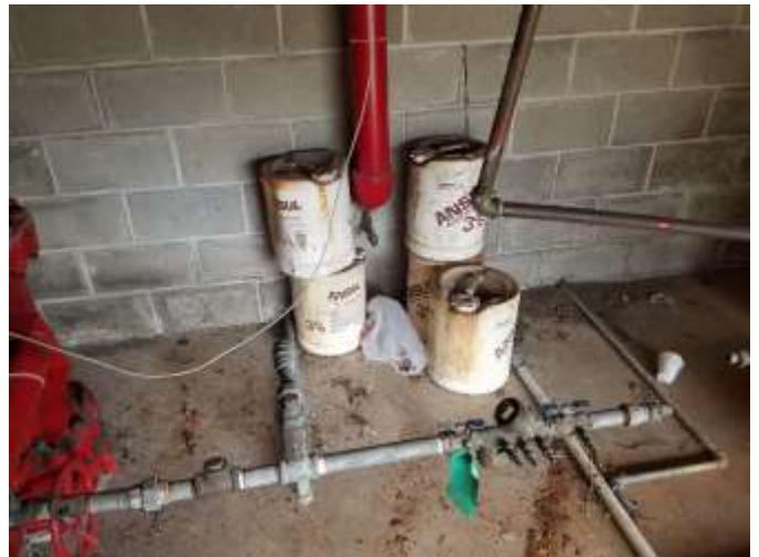
200. Sprinkler system equipment
