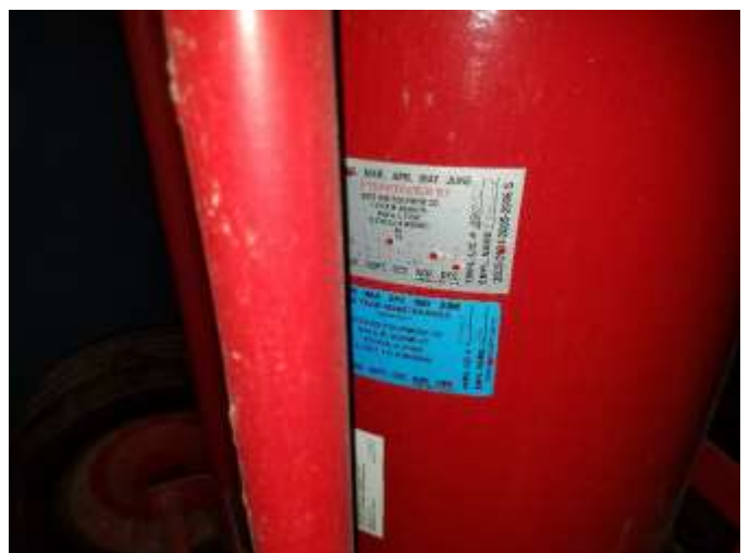
32. 150 lb AMEX wheel fire extinguisher
