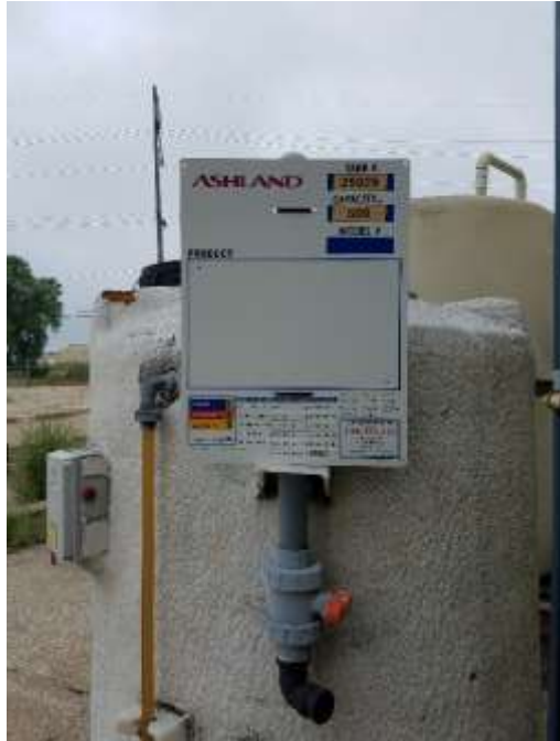
188. Ashland chemical storage tank 500 gallon
