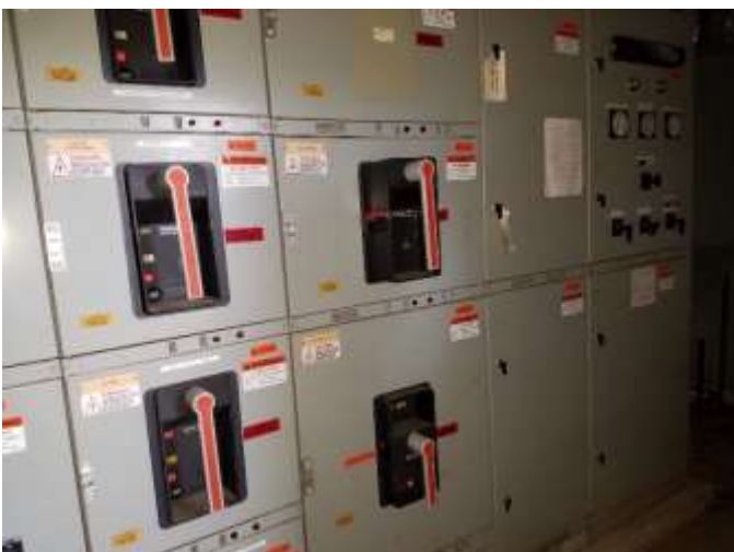
134. Inside control panel room
