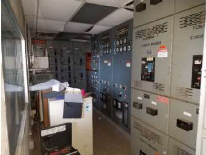
138. Inside control panel room
