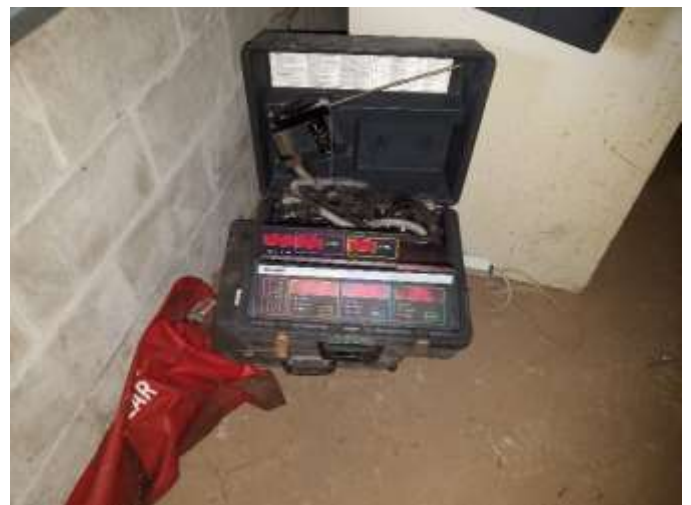
135. Inside control panel room
