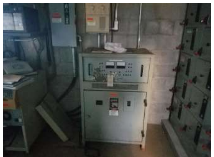
218. Generator control room
